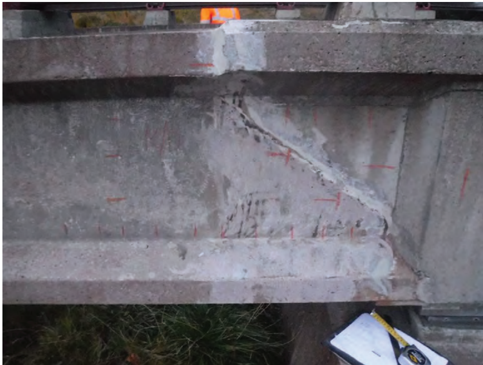
Plate 9 – General view of surface markings to Pier 22 Right Beam down
