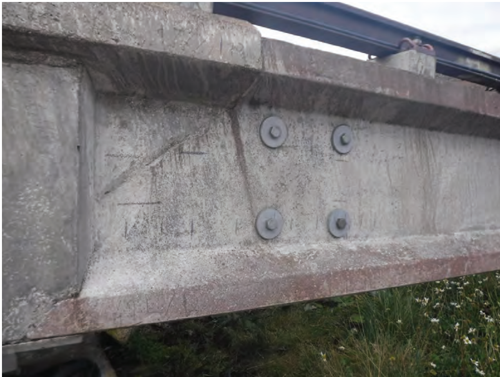
Plate 15 – General view of surface markings to Pier 49 Left Beam down
