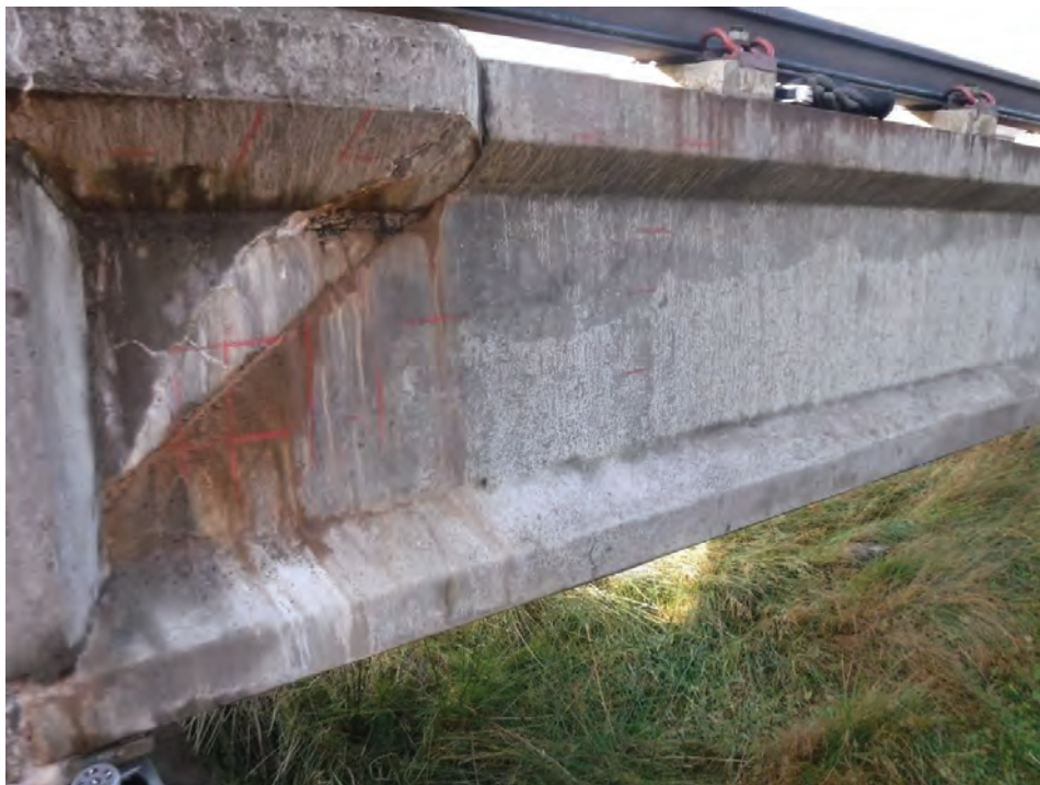
Plate 2 – General view of surface markings to Pier 9 Left Beam down.
