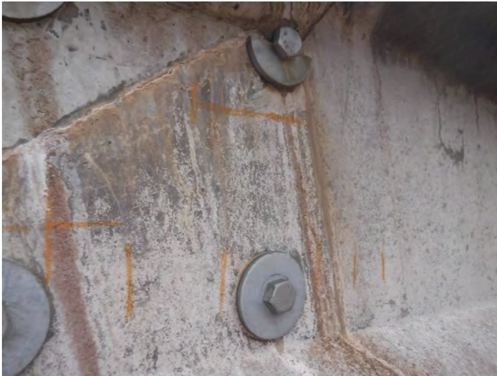
Plate 23 – General view of surface markings to Pier 53 Left Beam, Left support down
