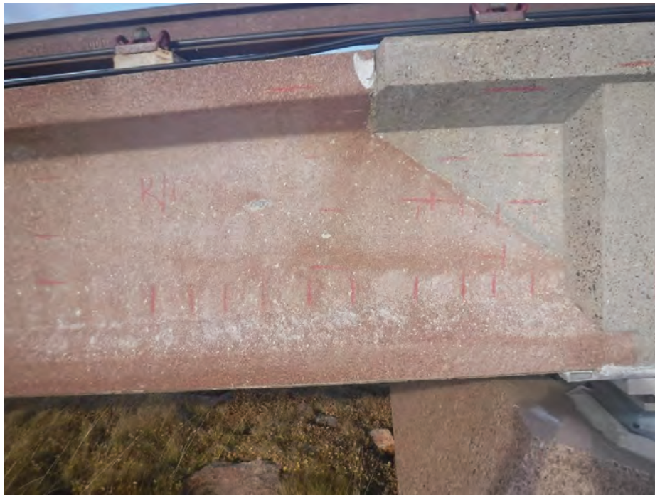
Plate 35 - General view of surface markings to Pier 69 Right Beam down
