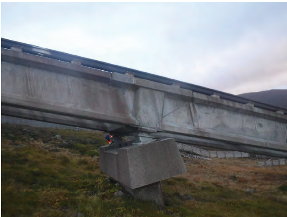
Plate 36 - General view of surface markings to Pier 69 Right Beam down
