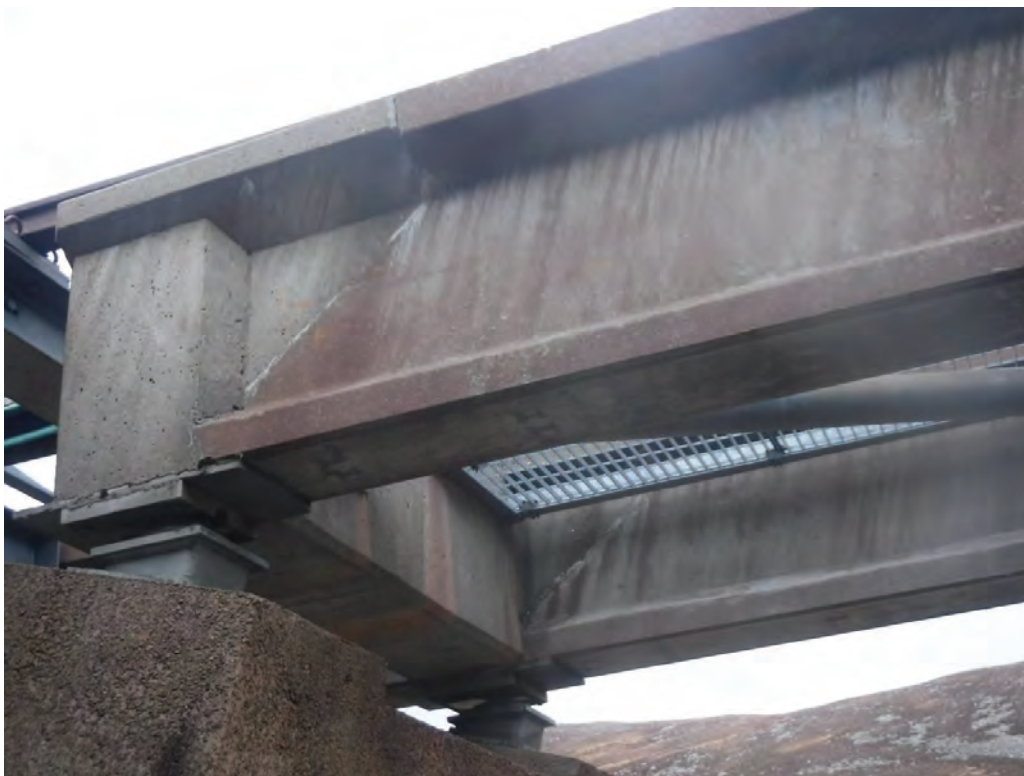
Plate 24 - General view of surface markings to Pier 53 Right Beam, left support up.
