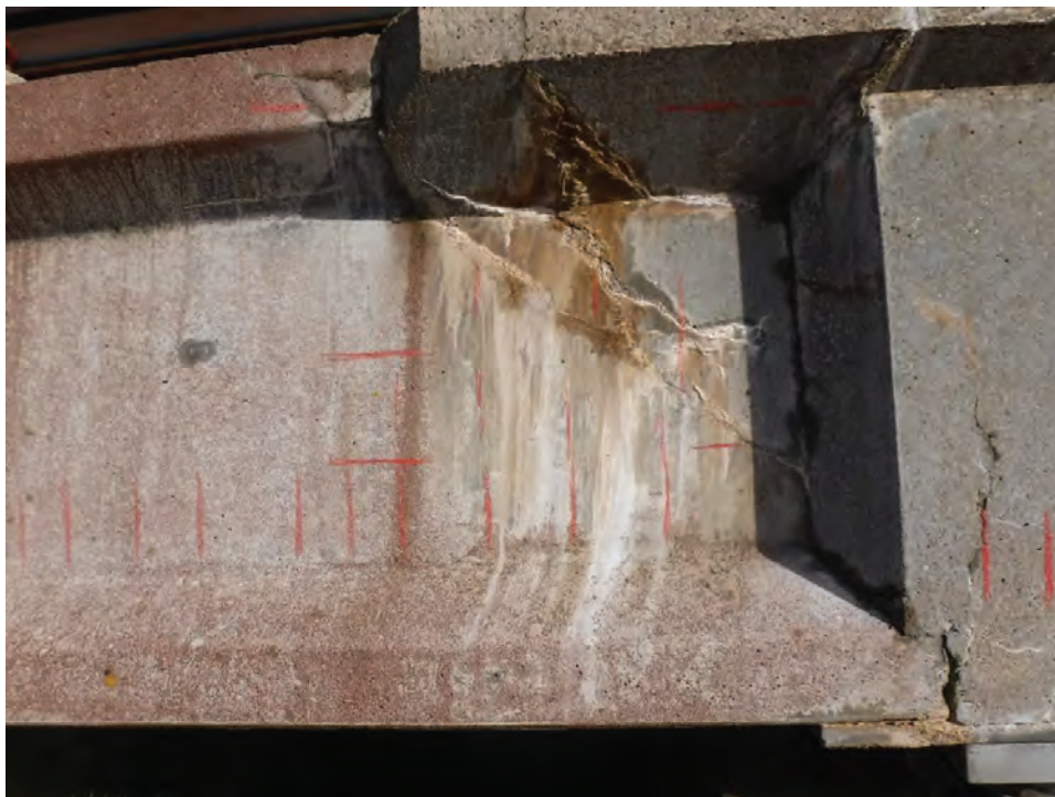
Plate 6 – General view of surface markings to Pier 9 Right Beam down
