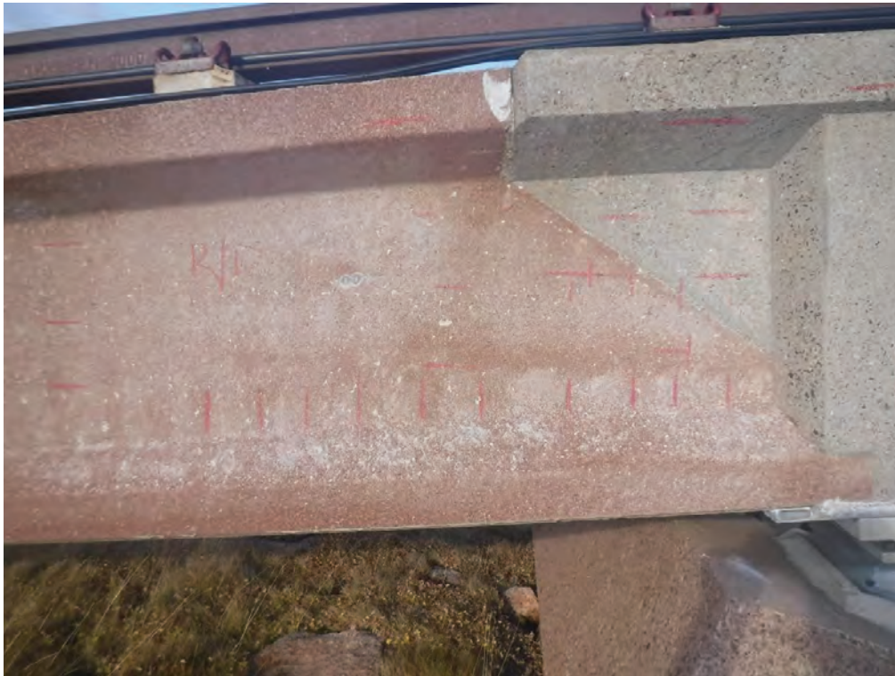
Plate 43 - General view of surface markings to Pier 80 Right Beam down
