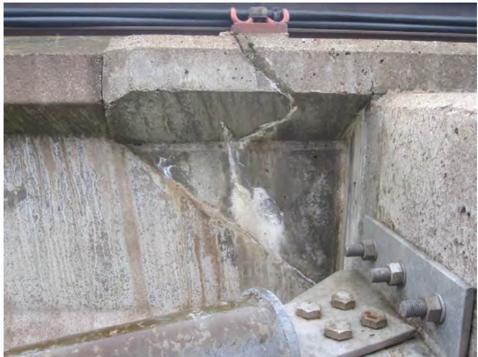
Figure 2-6 Cracking at a pier 9 (refer defect 1)
