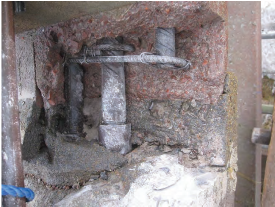
Figure 8 Breakout at pier 56 showing termination of T25 bar before the in-situ concrete interface
