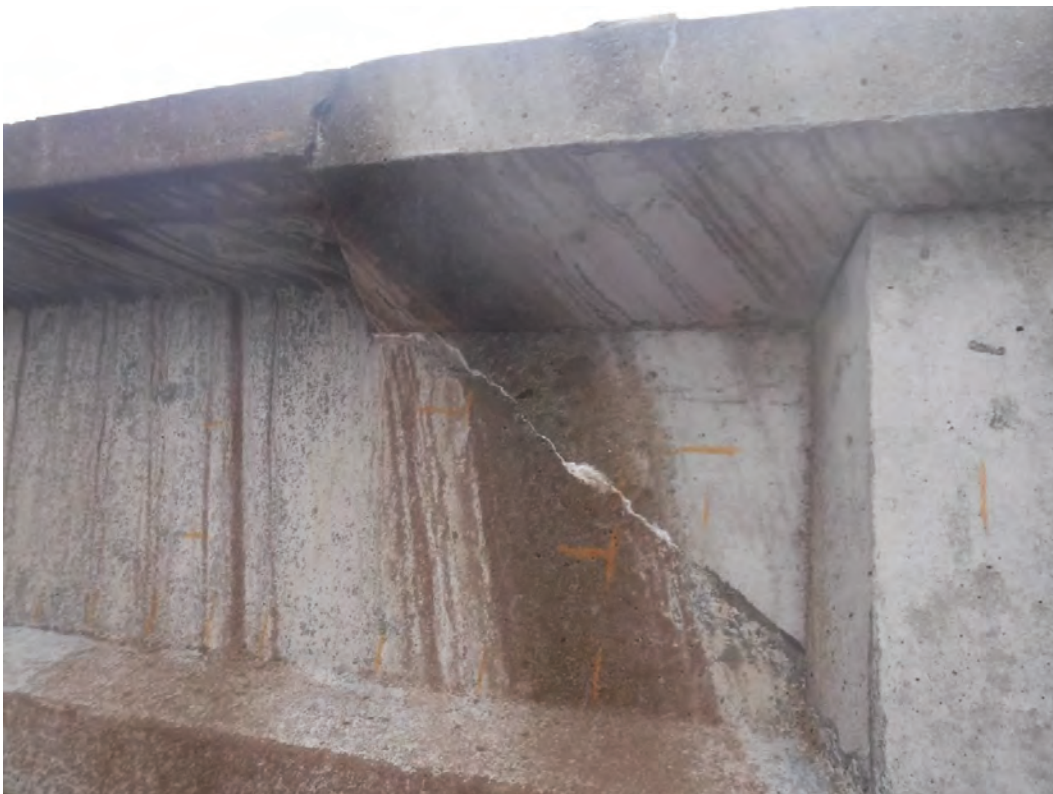
Plate 22 – General view of surface markings to Pier 53 Left Beam, left support up
