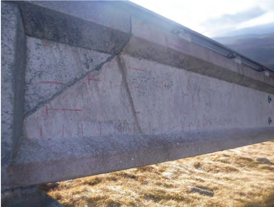
Plate 41 - General view of surface markings to Pier 80 Left Beam down
