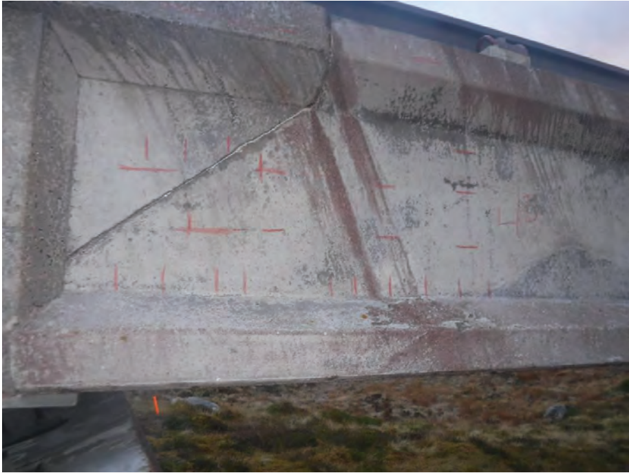
Plate 39 - General view of surface markings to Pier 69 Left Beam down
