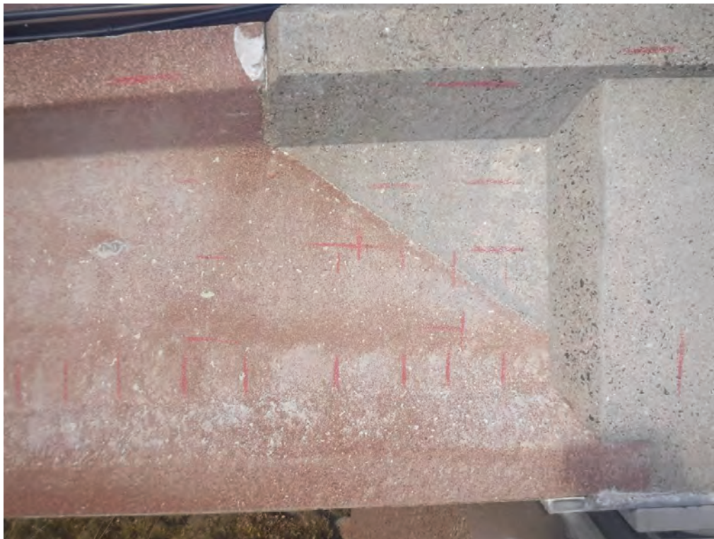
Plate 44 - General view of surface markings to Pier 80 Right Beam down
