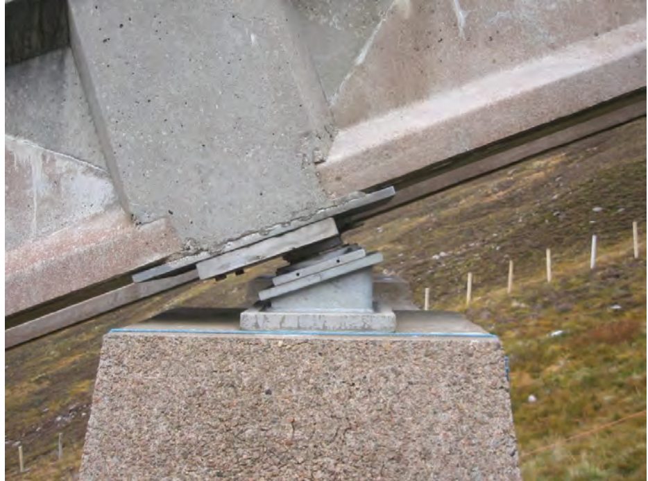
Figure 2-9 Bearing misalignment (refer defect 5)
