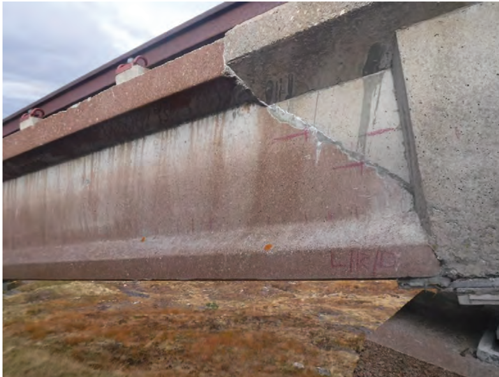
Plate 29 - General view of surface markings to Pier 54 Right Beam, left support down
