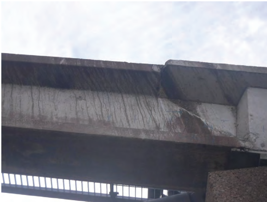
Plate 26 - General view of surface markings to Pier 54 Right Beam down
