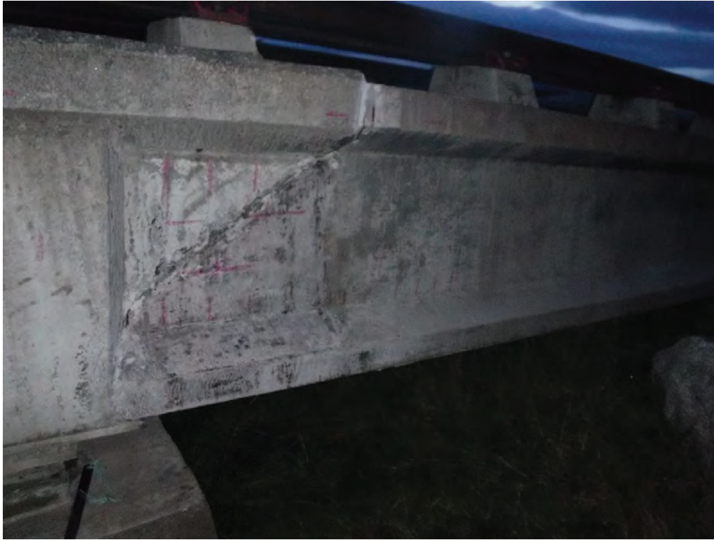
Plate 13 – General view of surface markings to Pier 22 Left Beam down
