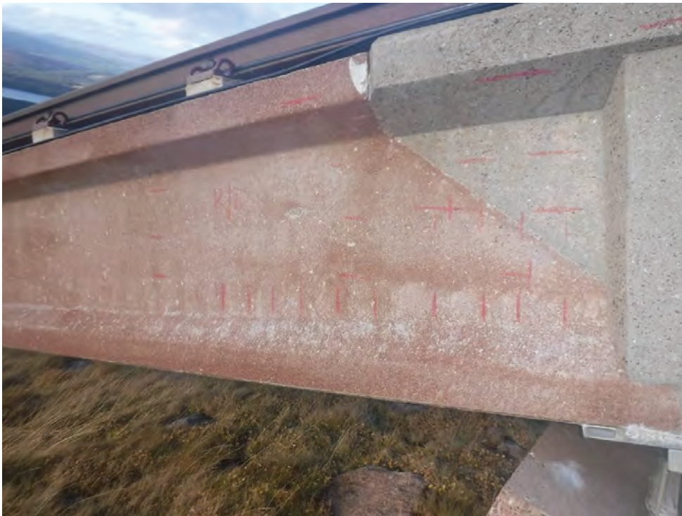
Plate 45 - General view of surface markings to Pier 80 Right Beam down
