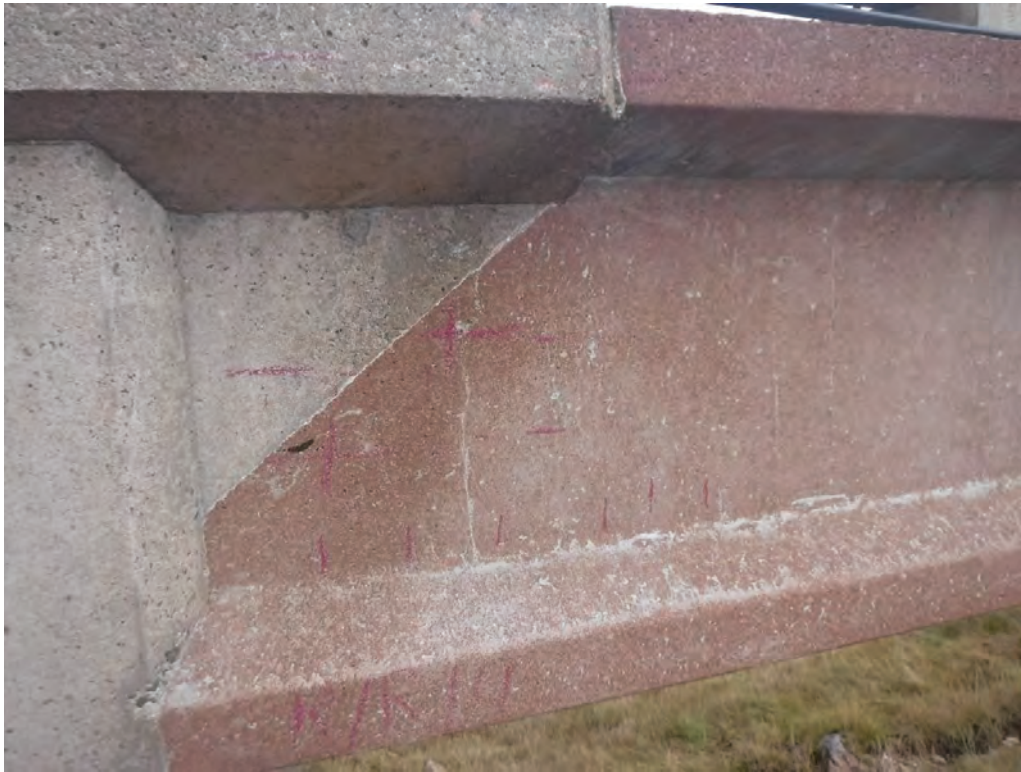
Plate 27 - General view of surface markings to Pier 54 Right Beam, right support up
