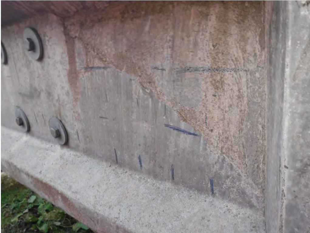
Plate 17 – General view of surface markings to Pier 49 Right Beam down
