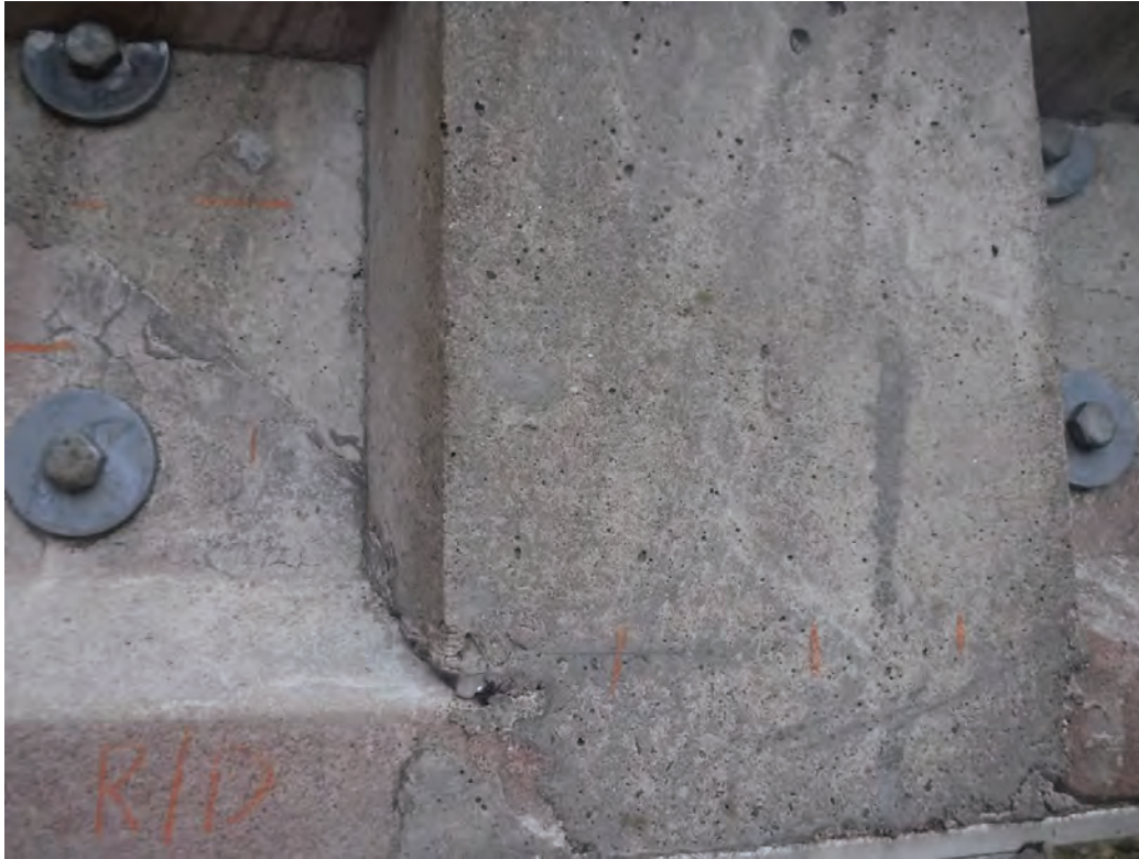
Plate 21 – General view of surface markings to Pier 51 Right Beam down
