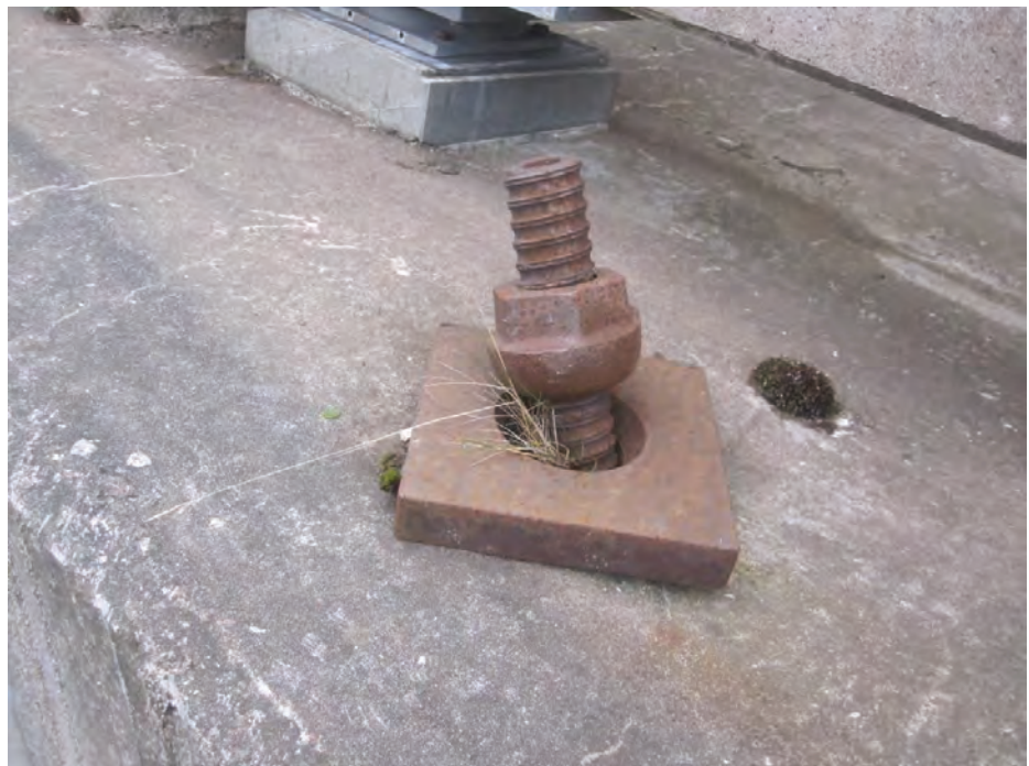
Figure 2-10 Loosened rock bolt in anchor block (refer defect 7)
