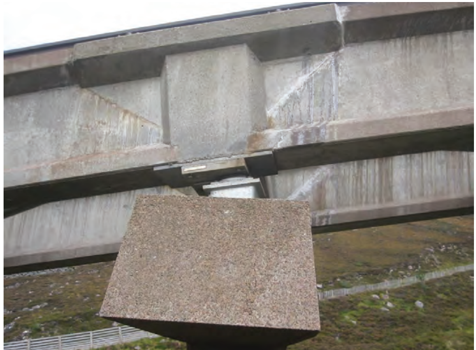
Figure 2-8 Typical crack leakage and bearing misalignment (refer defects 3 and 5)
