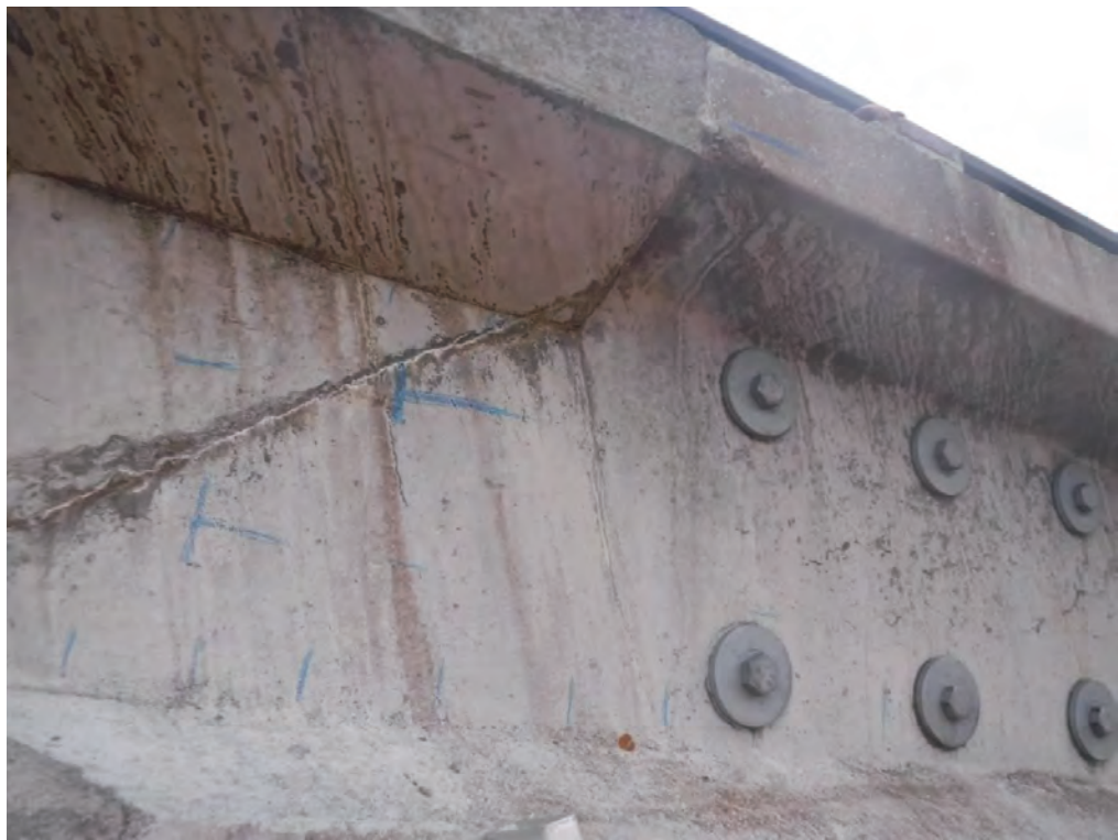
Plate 32 - General view of surface markings to Pier 56 Left Beam down
