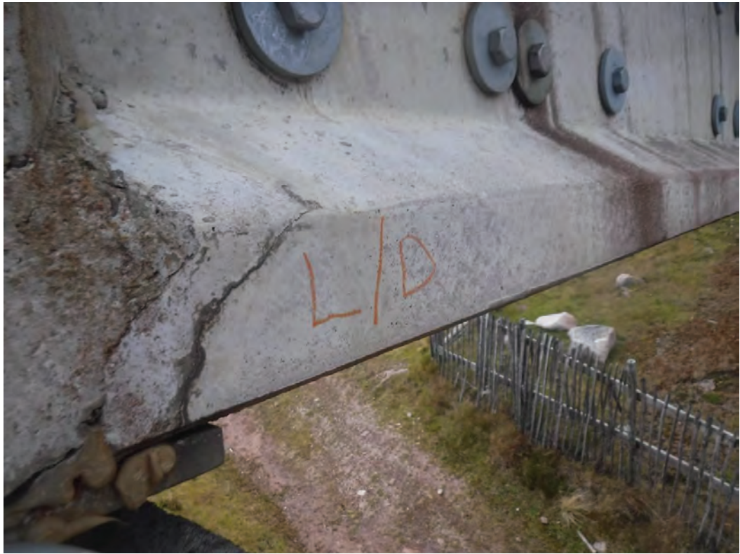
Plate 19 – General view of surface markings to Pier 51 Left Beam down
