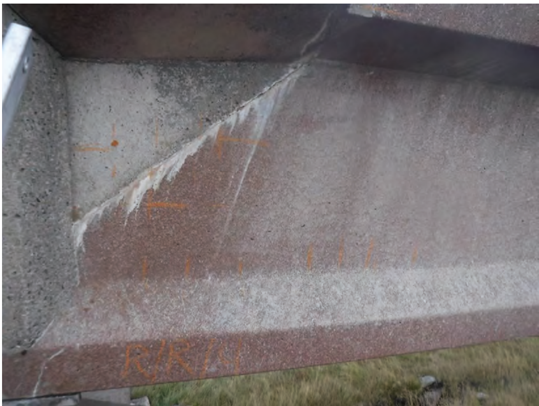
Plate 20 – General view of surface markings to Pier 51 Right, Beam right support up
